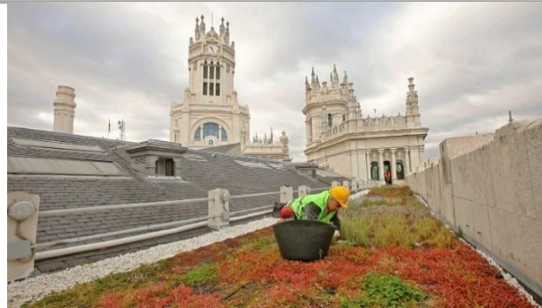
Figure 17 - Green roof installed over Madrid city hall.
